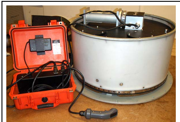
Valve in partially open position and shown with the Bambi Power Pack.
